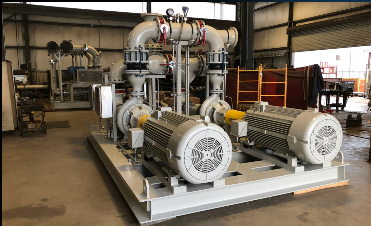
GE NRG Canal Pump Skid - Cooling Water Pump System
