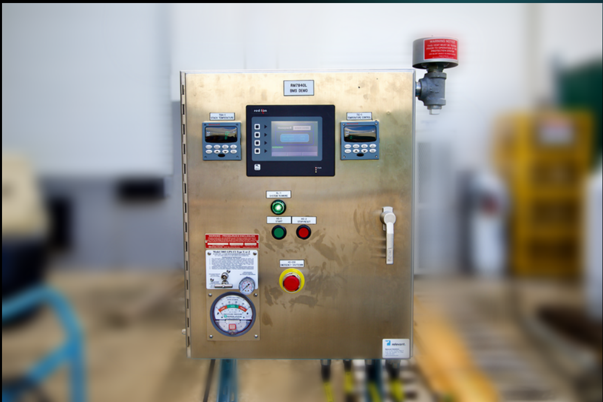
Burner Management Panel
